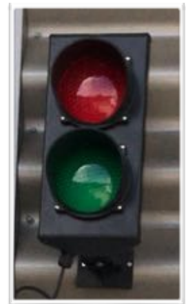
Exterior traffic light
