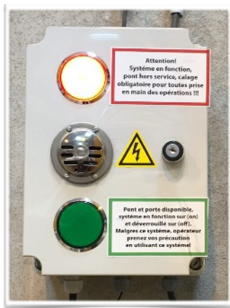
Interior Electric Control Box
